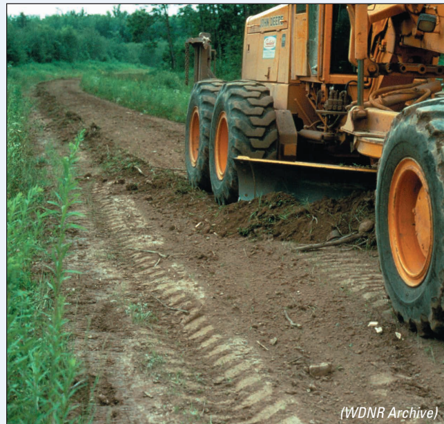
Figure 12-28: Maintaining woods roads helps prevent erosion. This grader is shaping the road surface so that water runs off properly.
