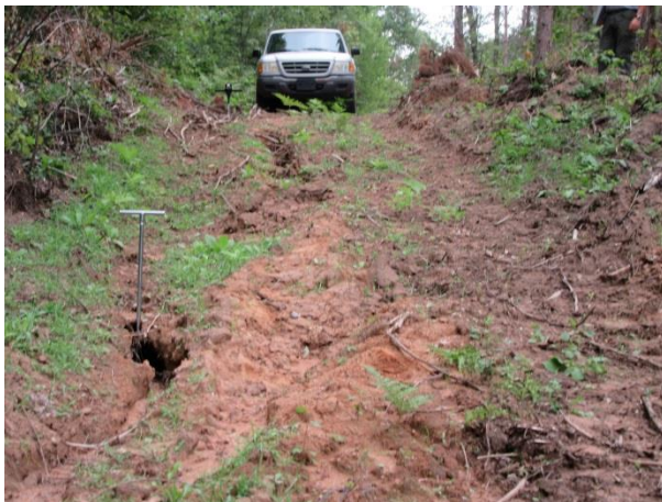
Figure 2. Gully on a forest road system. Lack of water control structures, led to channelized run-off forming gullies that have active erosion.
