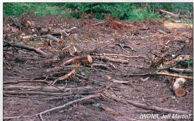
Figure 16-21: Retaining slash on skid trails is an effective way of reducing soil compaction and rutting from use of heavy logging machines.
