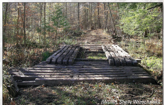
Figure 12-6: Timber mats provide an easy and cost-effective option for temporary stream crossings.
