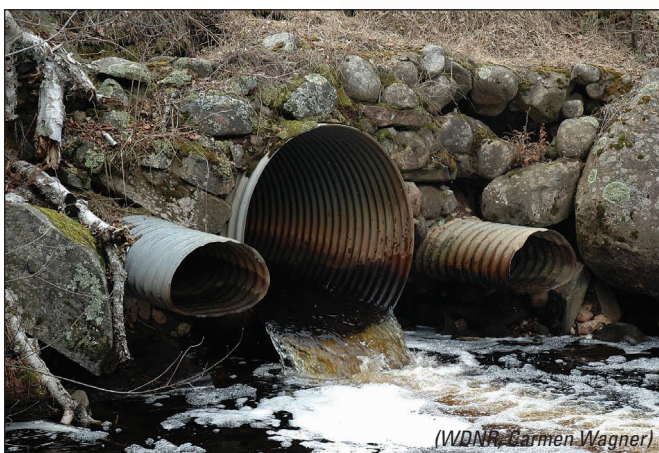
Figure 12-5: This stream crossing is undersized and perched, preventing fish movement upstream.
