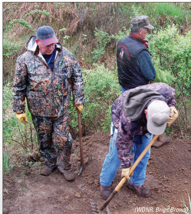
Figure 18-7: Trail construction should consider invasive plants. The honeysuckle shrub adjacent to this trail and other invasive plants may spread or invade new areas dues to the disturbance.
