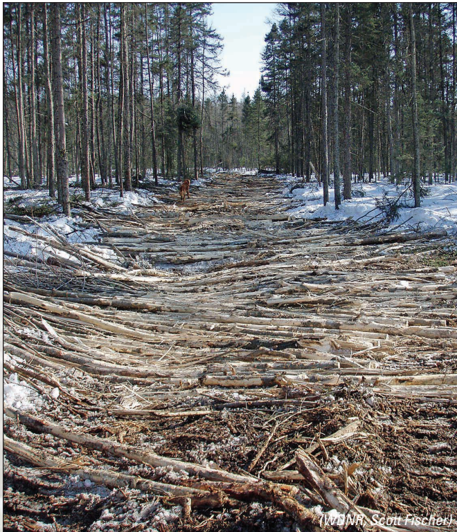
Figure 5-17: To help support equipment and minimize rutting, slash can be used as a temporary wetland crossing. See Chapter 12: Forest Road Construction and Maintenance for more information about this practice.
